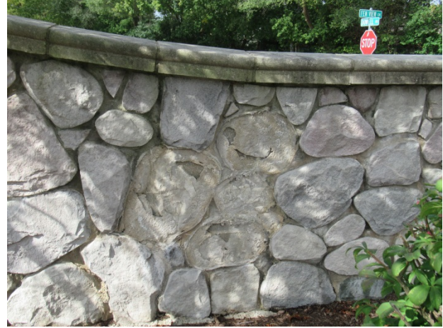
Missing stone veneer
